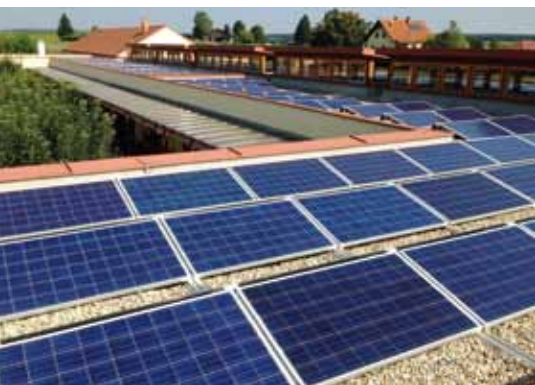
■ Photovoltaikanlage in Strem
